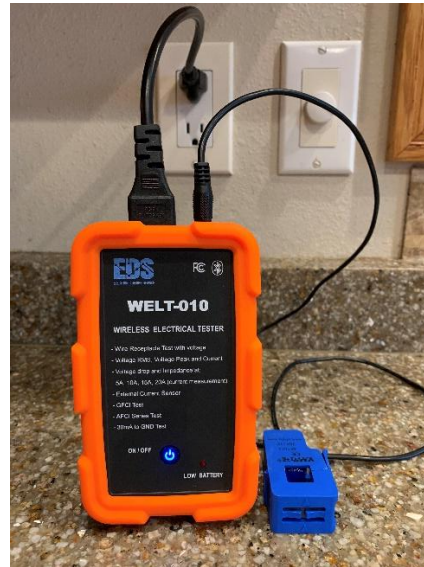
Figure 4 Voltage, Voltage Drop Measurements, Socket Monitor, GFCI and AFCI Tests
